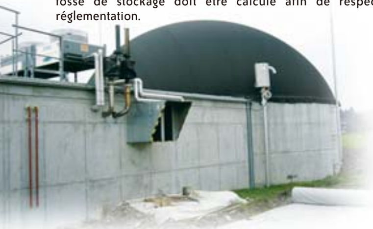
Photo 5 : Post-digester (source Aile)
